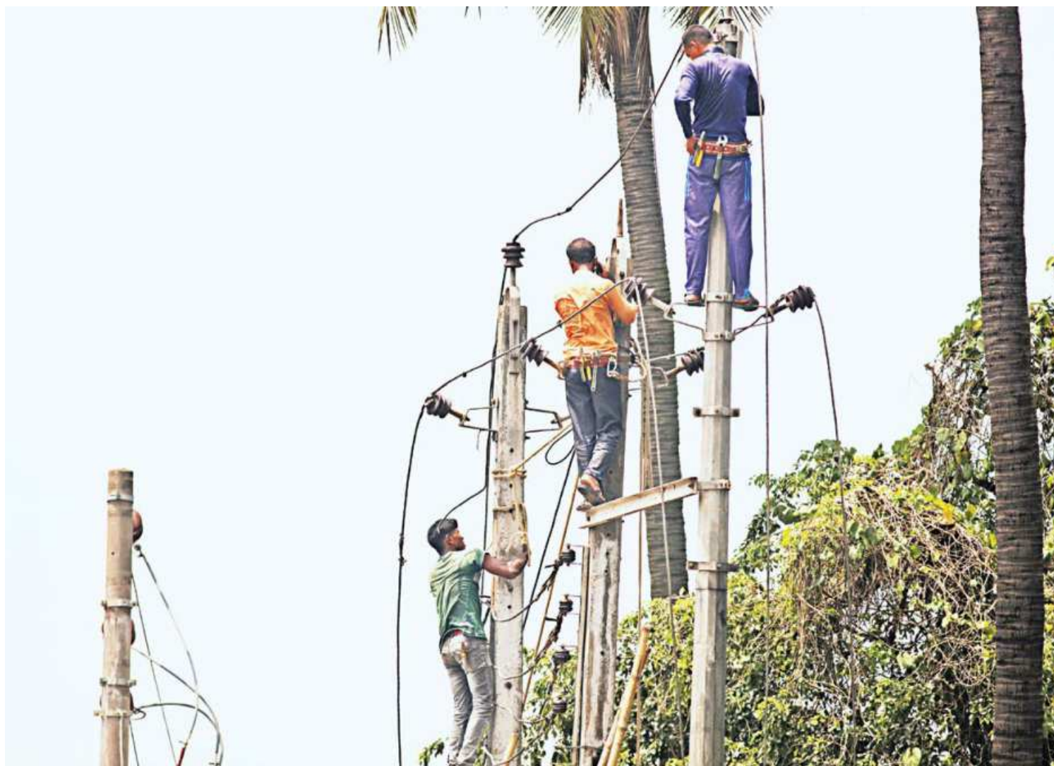
A group of Dhaka Power Distribution Company staffers were spotted yesterday fixing electrical poles at Kalyanpur, opposite the Khaleque Service Station. Though the task carries risk of fatality from electrocution, none of the workers seem to be wearing any protective gear, an issue persists despite repeated condemnations from activists and coverage in press.
