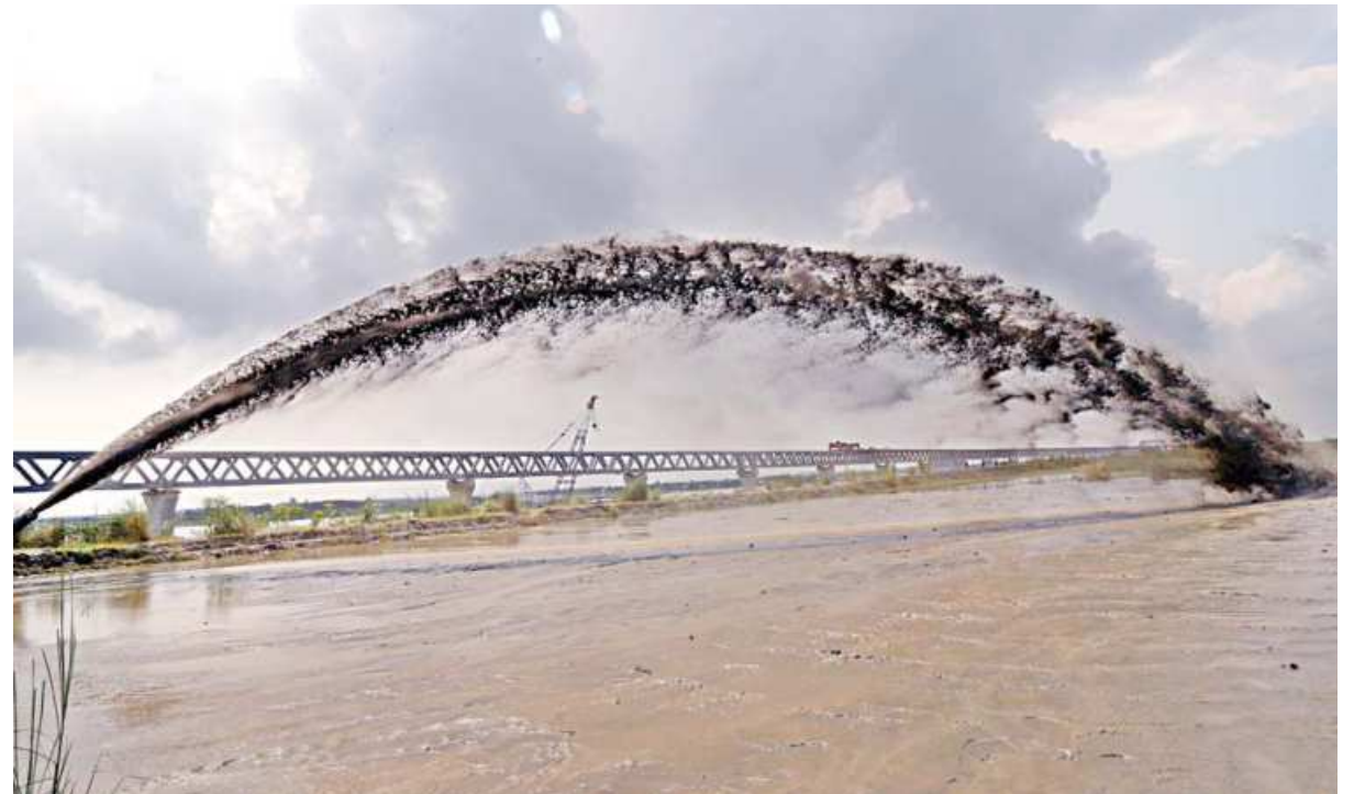
Silt dredged from the Padma being dumped in an area close to the Padma bridge yesterday to restore navigability of ferries between Shimulia and Kathalbari ferry terminals. Ferry services have been suspended there for a week, forcing vehicles to make a detour and use the Aricha-Doulatdia ferry terminals.
