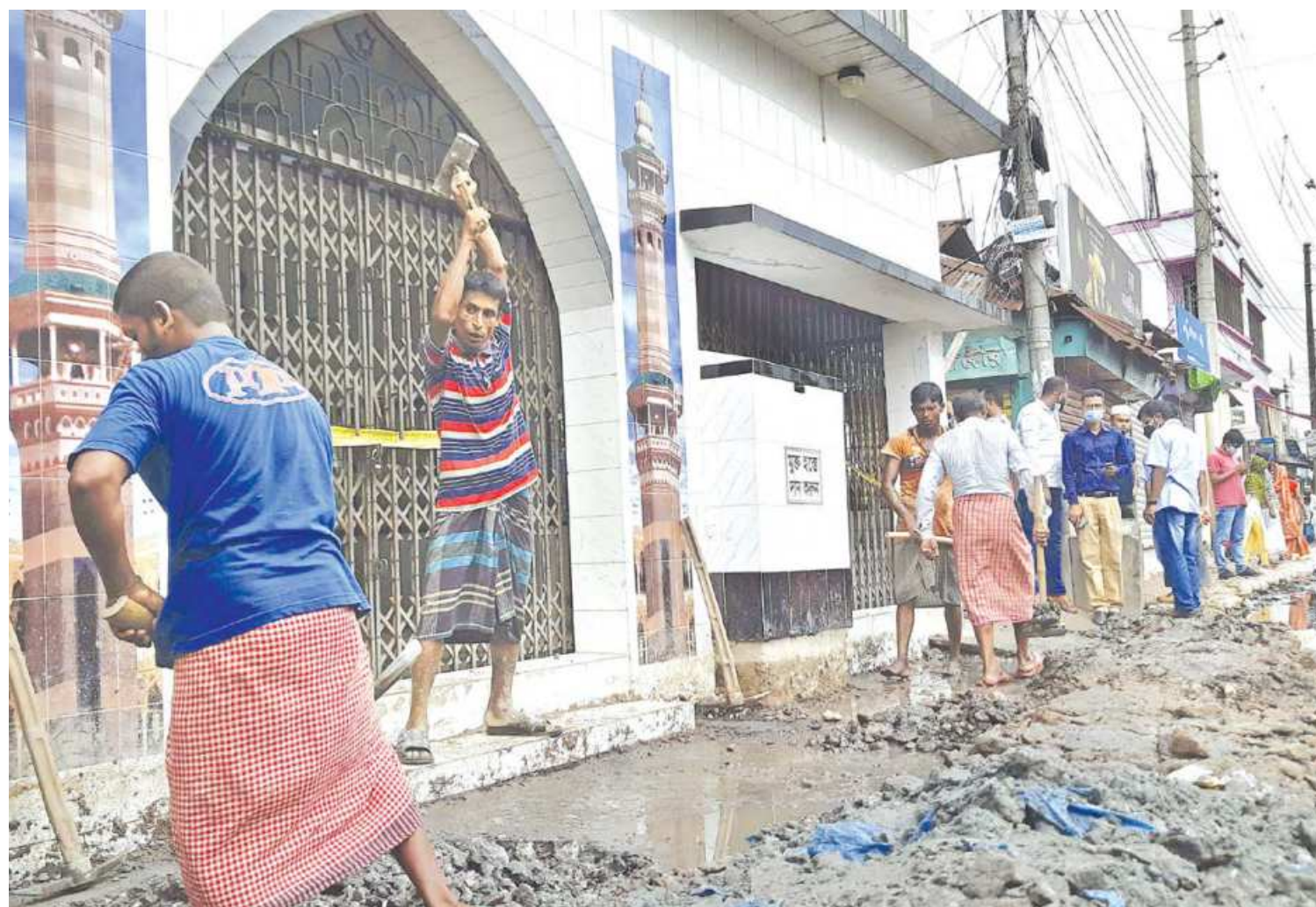
Workers hired by Titas Gas dig the ground in front of Pashchim Talla Baitus Salam Mosque in Narayanganj yesterday. Later in the day, a pipeline of Titas was found there. A fire at the mosque on Friday night, believed to be caused by gas from a leaking pipeline, killed 27 people and burnt a dozen others.
