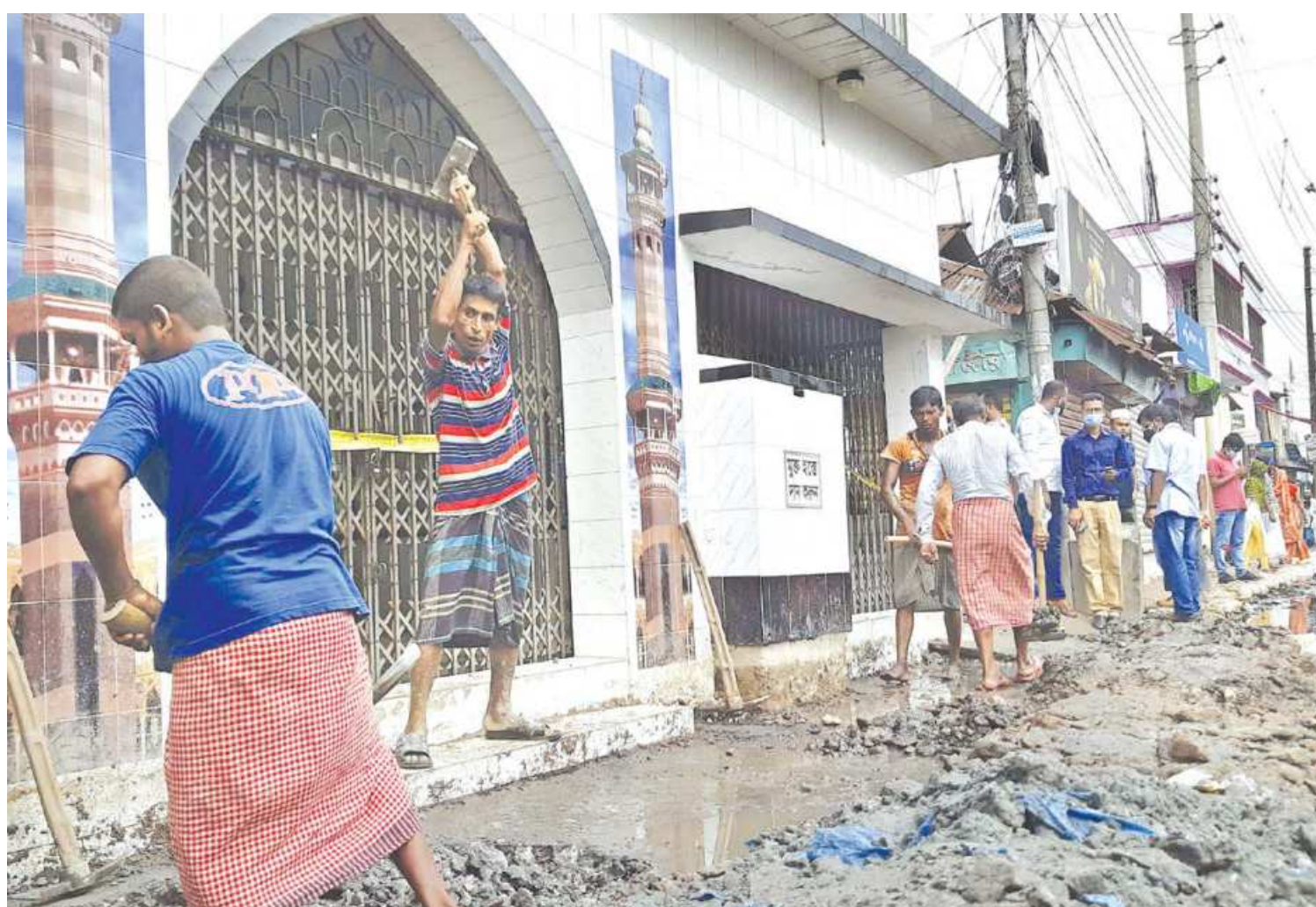
Workers hired by Titas Gas dig the ground in front of Pashchim Talla Baitus Salam Mosque in Narayanganj yesterday. Later in the day, a pipeline of Titas was found there. A fire at the mosque on Friday night, believed to be caused by gas from a leaking pipeline, killed 27 people and burnt a dozen others.
