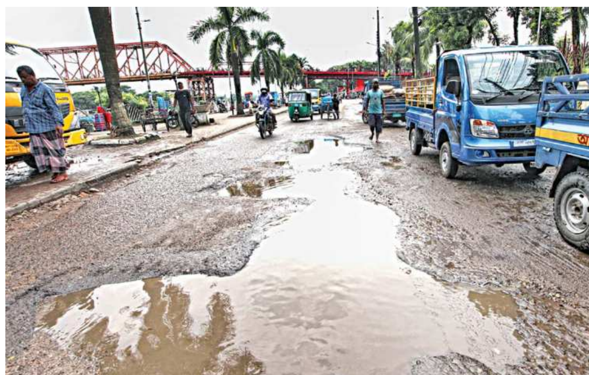
Everyday, around 2,000-5,000 vehicles pass through this strip at Sylhet's Circuit House area's Kali Ghaat road. In spite of its importance, the road has remained in an awful state for a long time. To add to this, a few hundred trucks are constantly parked on it, even though it's under a VIP zone. The same can be said about many other roads at the city's Bandar Bazar, Surma Point and more. Starved of repair works, the streets have become a cause for concern for commuters, even moreso during rainy seasons, when the suffering increases manifold. This photo was taken yesterday.
