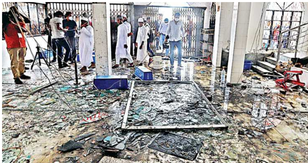
The ground floor of the mosque in Narayanganj's Talla area is littered with warped blades of ceiling fans, charred remains of human flesh and prayer rugs, shards of glass and debris. At least 20 people have died in Friday's explosion there.
