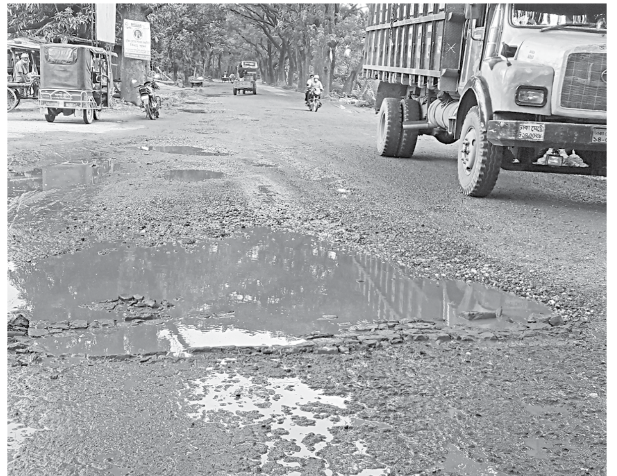
A truck passes by a large pothole on Jhenidah-Kaliganj highway. The photo was taken recently.
