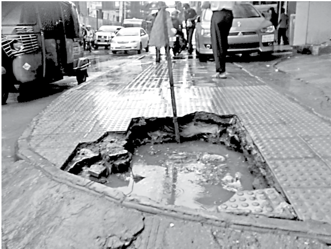
On the footpath stretching from Karwan Bazar to Farmgate, at least seven to eight such craters have been created which turn into dangerous puddles after rain. With the capital going back to its busy self gradually, these would only bring more suffering to pedestrians. The photo was taken yesterday.
