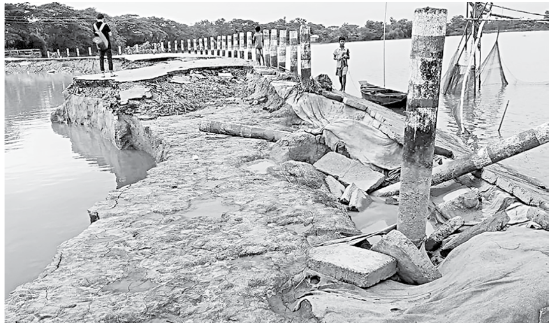
Thanks to three waves of floods in two months, this is what many parts of Sunamganj-Chhatak road now look like.
