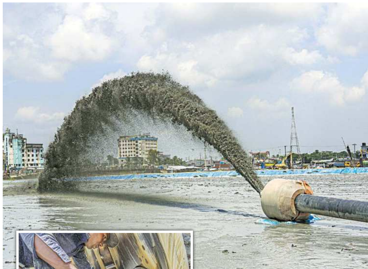
Dredging of the Karnaphuli river resumes after being suspended for a long time because of the pandemic. But the challenge is discarded plastic goods at the bottom of the river clogging the machine in about every 15 minutes. Inset, mechanics removing plastic bags from a cog yesterday.
