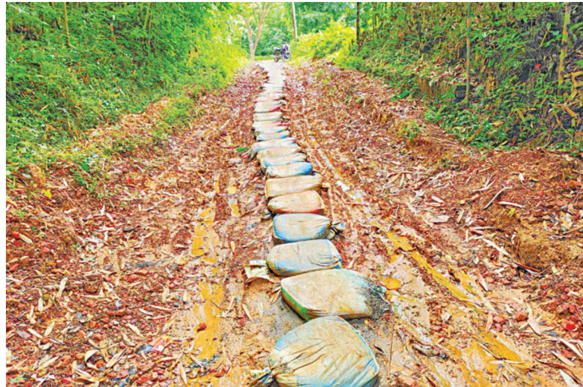
Construction of the 780m-long Deopara-Shatak road in Habiganj's Nabiganj upazila was about to be completed in May 2020, but it did not happen due to various irregularities by the contractor. Such a dilapidated state of the road has long been affecting the communication of people in nearby areas. PHOTO: MINTU DESHWARA
