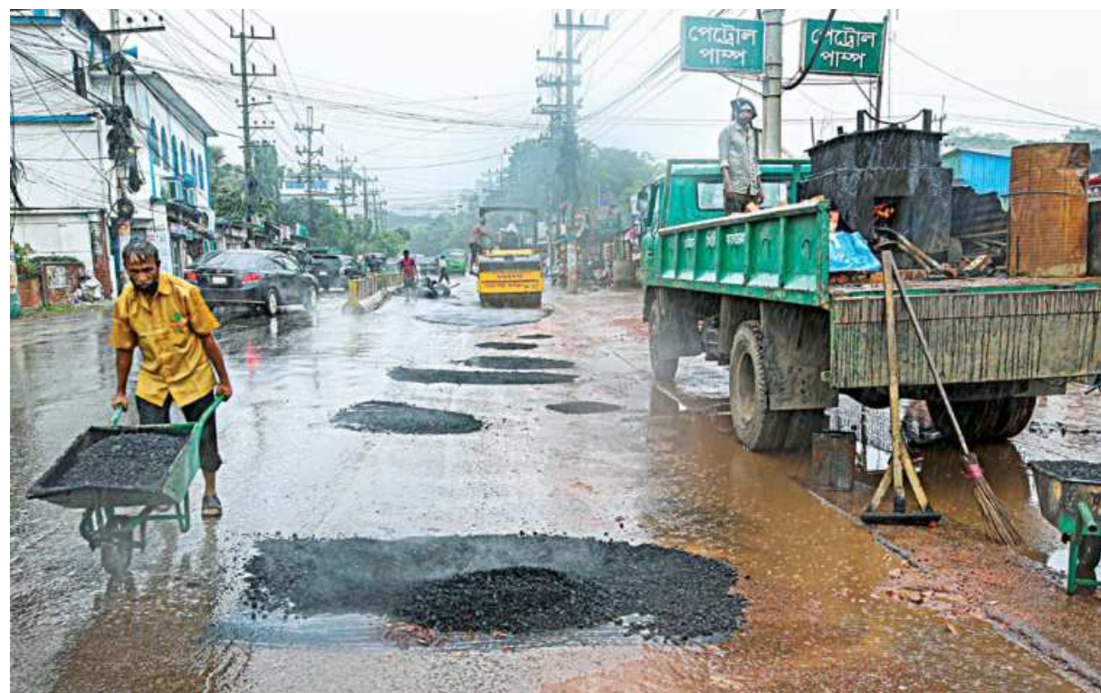
Despite rain, workers of Chattogram City Corporation were seen busy repairing this road at the port city's Khulshi area. However, all their hard work might go to waste, as the Bitumen -- the material used for forming roads -- can be ineffective in holding the surface together if it is exposed to water during application. As a result, it will not be surprising if the potholes return after a few months. The photo was taken on Wednesday. PHOTO: RAJIB RAIHAN
