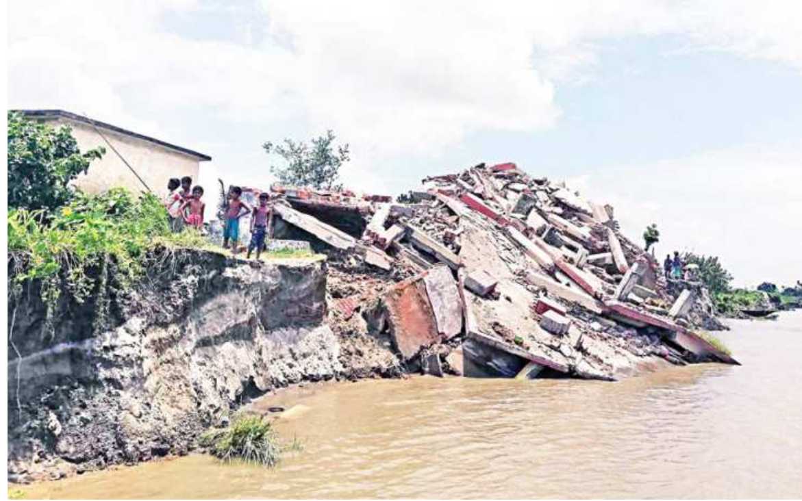
Paiksha Majhail Government Primary School in Tangail lies in ruins after being ravaged by the Jamuna. Many school buildings in the district have suffered a similar fate due to river erosion and ongoing floods. The photo was taken recently.
