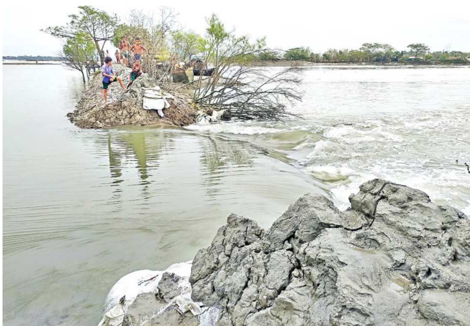
Water rushing towards Pratapnagar union in Satkhira's Assasuni upazila after a dam collapsed due to heavy pressure of water on Thursday. The dam was damaged during cyclone Amphan, but authorities took no steps to repair it in the last few months. The photo was taken yesterday.
