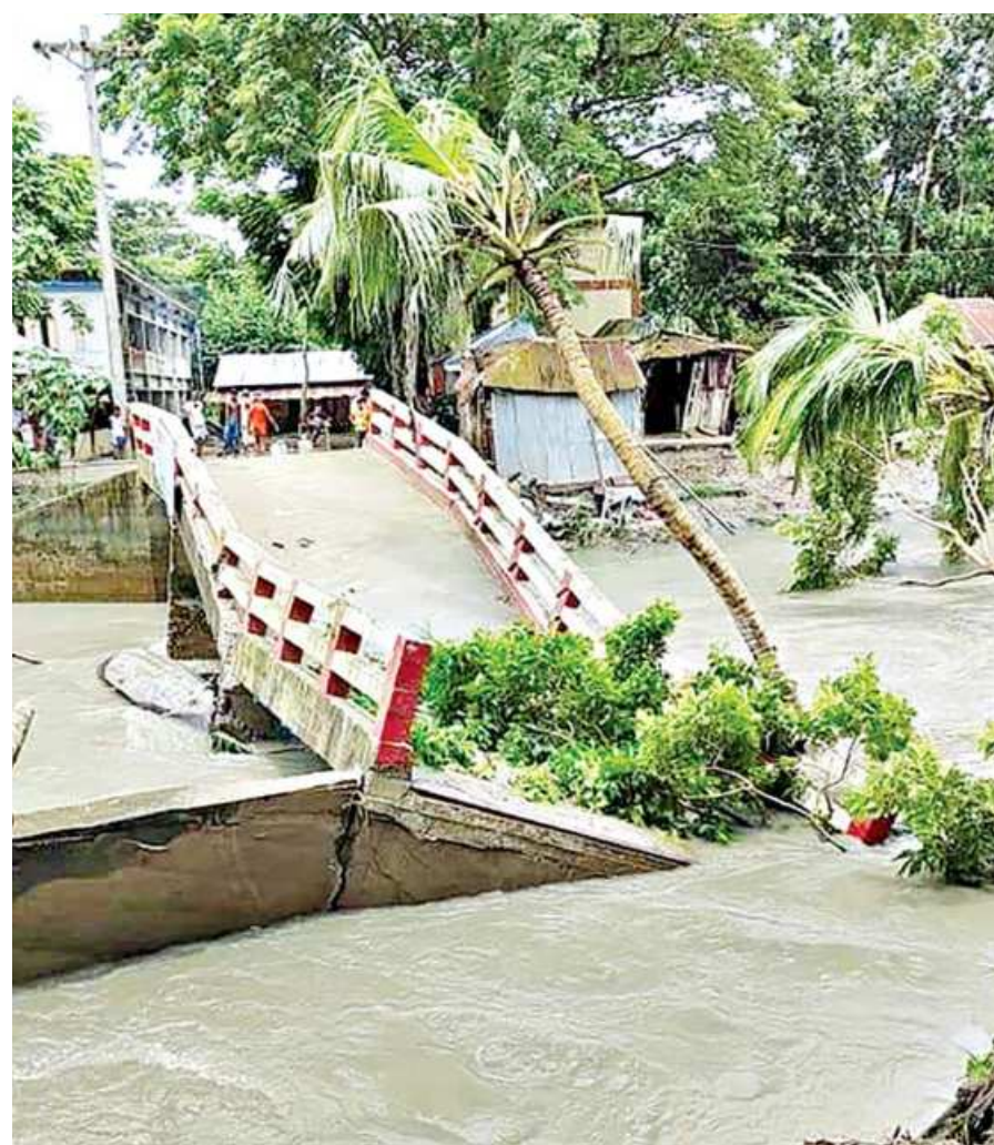
A bridge gives way to rush of floodwaters and high tide in Mehendiganj upazila of Barishal district, causing sufferings to locals. The bridge connects Ullania union and Hazirpur.
