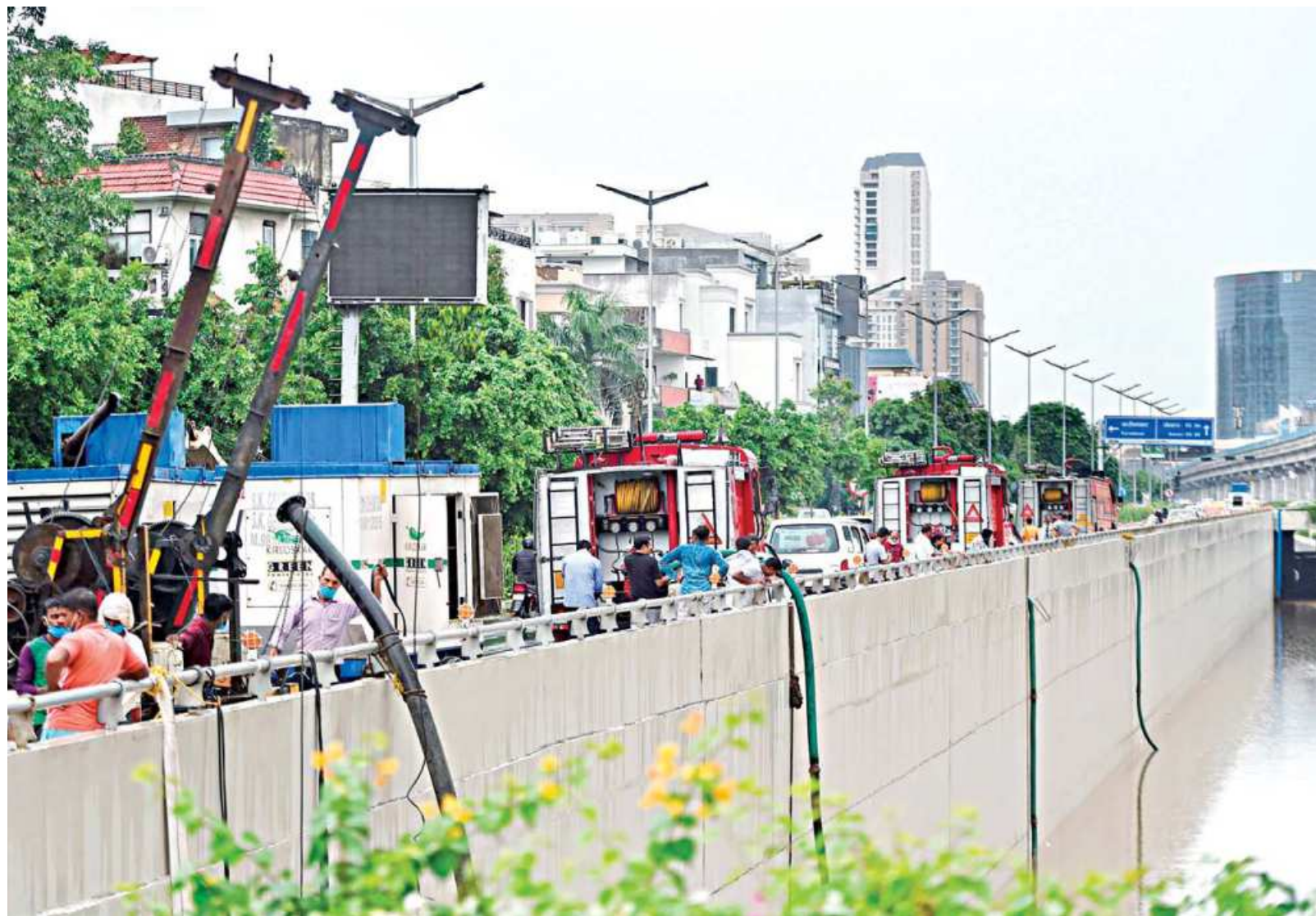
Fire crew members and municipal workers make a concerted effort to pump out water from a flooded road underpass following monsoon rainfalls in Gurgaon on the outskirts of New Delhi, India yesterday.
