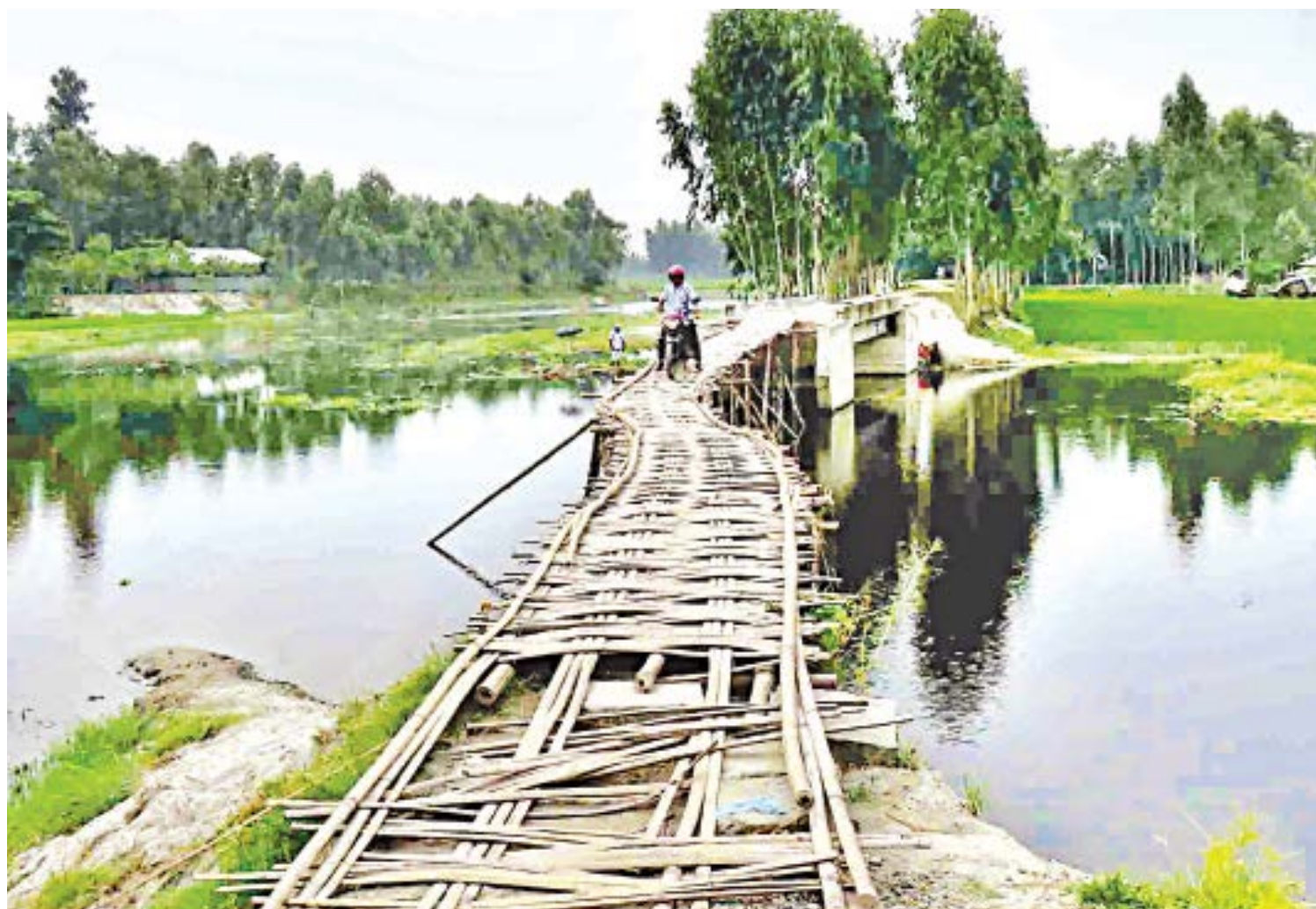
The rush of floodwater washed away the approach road to this bridge in Char Islu village of Rangpur's Gangachara upazila. Desperate for a usable bridge, the locals did not bother to wait for it to be mended. They made it passable by building an approach road out of bamboo poles and fences. The photo was taken yesterday.
