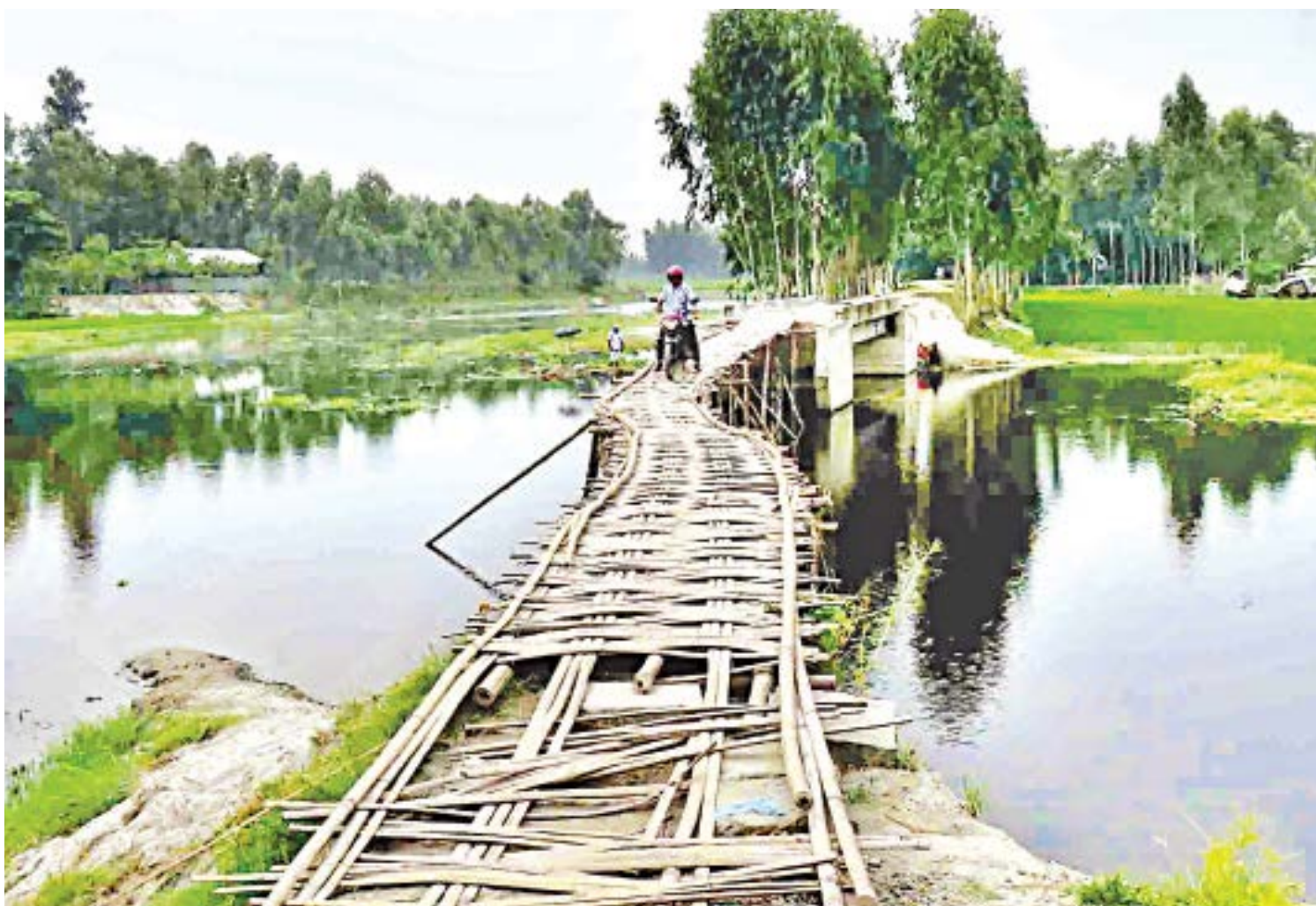
The rush of floodwater washed away the approach road to this bridge in Char Islai village of Rangpur's Gangachara upazila. Desperate for a usable bridge, the locals did not bother to wait for it to be mended. They made it passable by building an approach road out of bamboo poles and fences. The photo was taken yesterday.
