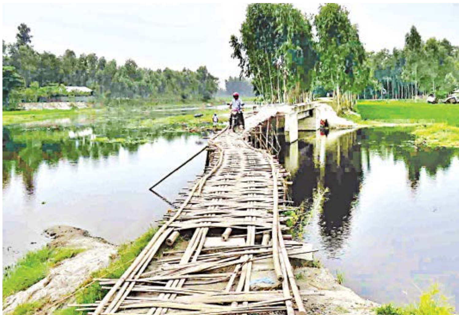
The rush of floodwater washed away the approach road to this bridge in Char Islu village of Rangpur's Gangachara upazila. Desperate for a usable bridge, the locals did not bother to wait for it to be mended. They made it passable by building an approach road out of bamboo poles and fences. The photo was taken yesterday.
