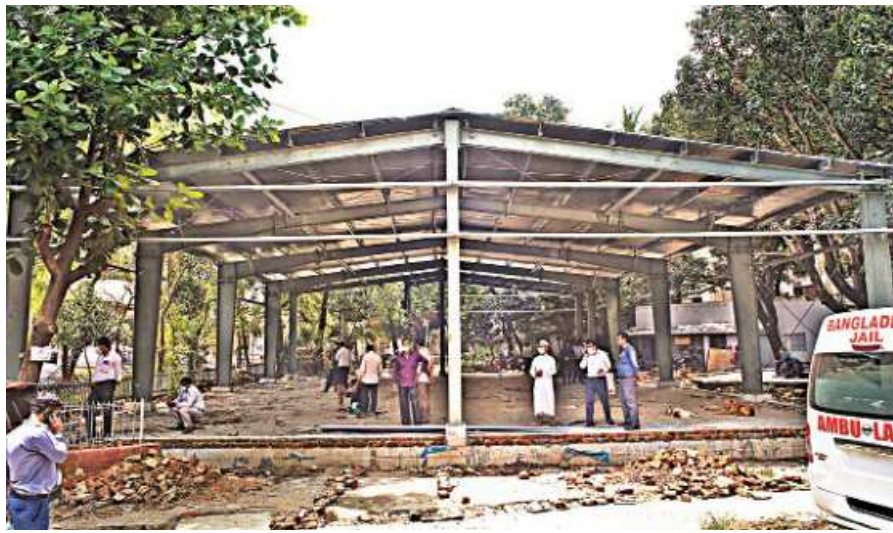
Once completed, this 7,500 sq ft steel structure will help ease long queues and serve additional patients. The photo was taken last week.
