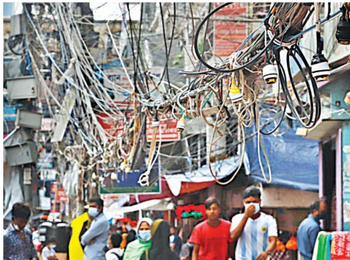
An array of lightbulb sockets hang on a tangle of wires outside the Muktijoddha Super Market in the capital. Roadside hawkers in front of the market use electricity from inside the market by connecting power cables, paying a daily "fare" of Tk 40-50, locals said. Not only is this practice illegal, but the exposed livewire connections on the sockets poses a constant risk of electrocution, especially in rainy weather.
