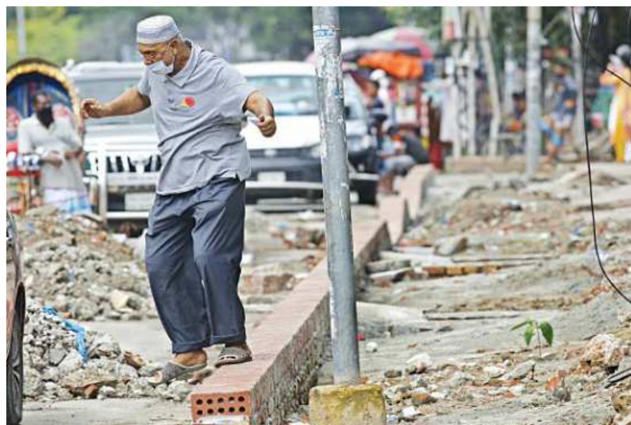
For over a month, footpaths on the capital's Satmasjid Road have remained in this condition, leaving pedestrians no other option than to hop, skip and jump over debris. City corporation workers are doing such renovation work in many parts of Dhanmondi, which locals say are in a haphazard manner.
