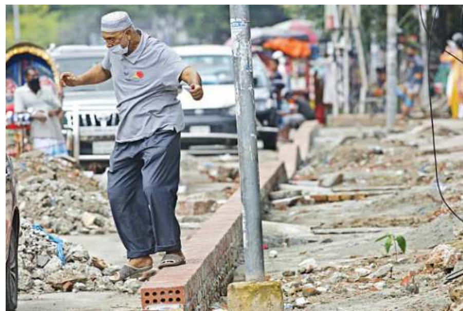
For over a month, footpaths on the capital's Satmasjid Road have remained in this condition, leaving pedestrians no other option than to hop, skip and jump over debris. City corporation workers are doing such renovation work in many parts of Dhanmondi, which locals say are in a haphazard manner.
