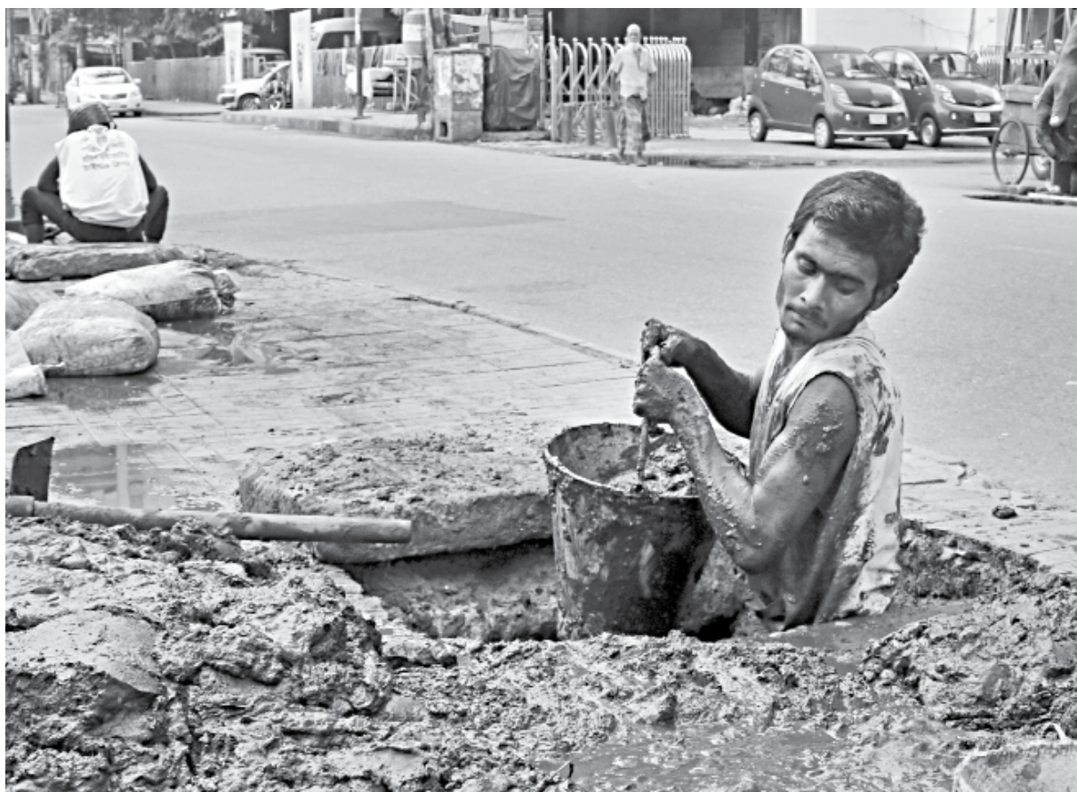
City corporation workers remove sludge from drains on the capital's Kazi Nazrul Islam Avenue, with no safety gear. The lack of protective covering exposes them to harmful pathogens and toxic fumes, which may lead to severe health complications. This photo was taken on Friday.
