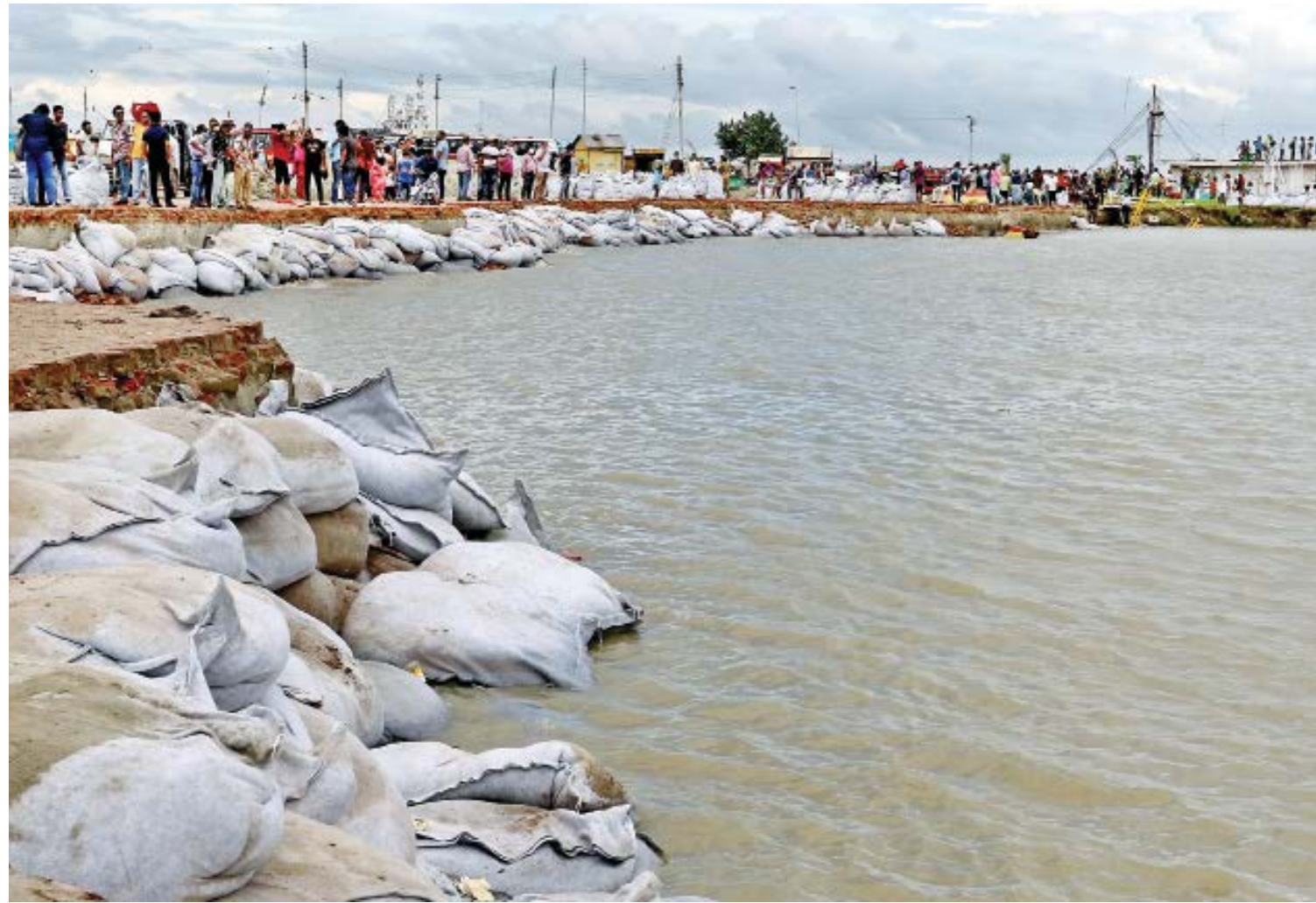
The approach road to the ferry pontoon-4 at Shimulia of Munshiganj went under water due to the erosion by the Padma yesterday morning. Geo-bags are being dumped there to stop the erosion. Another road to a pontoon was devoured by the river before Eid. The erosion of the bank is disrupting ferry services.
