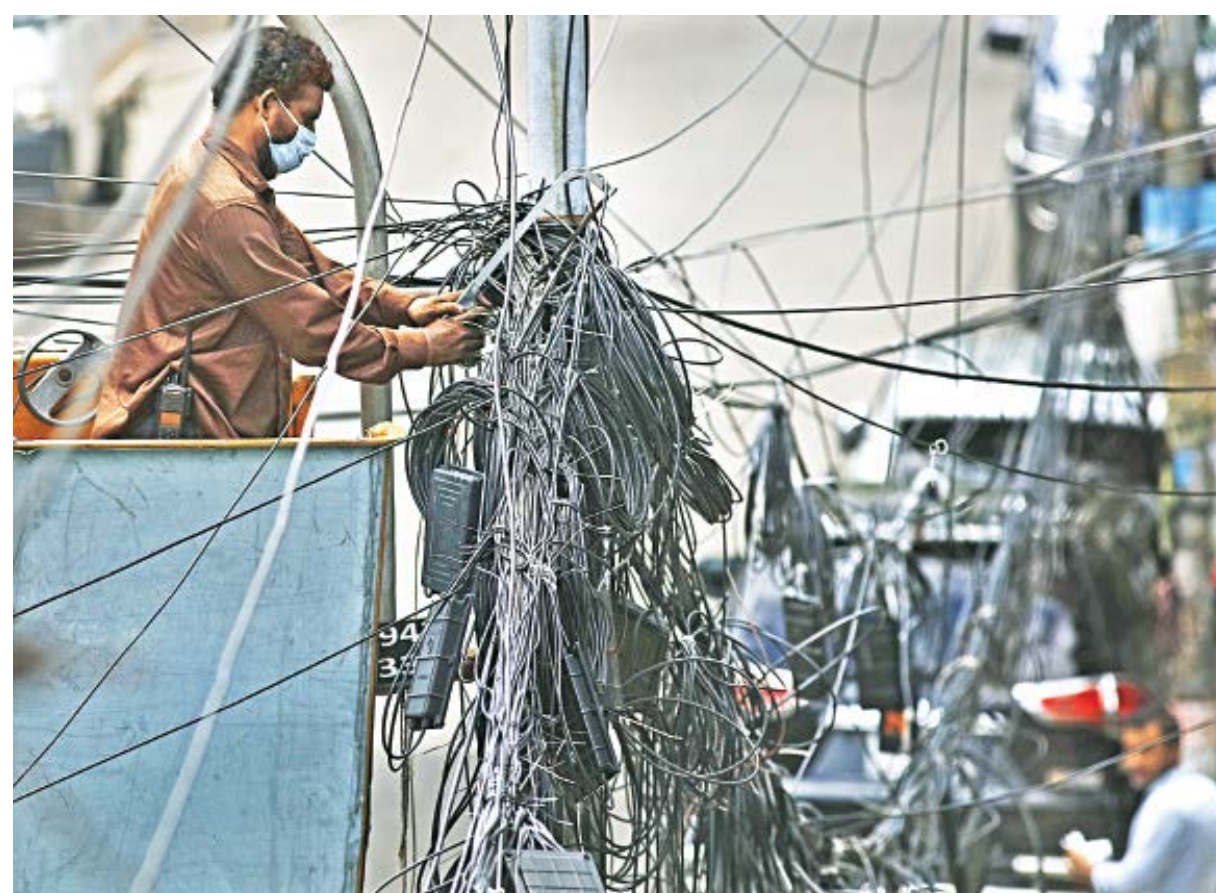
Riding a crane-lifted work box, a Dhaka North City Corporation staff uses a hacksaw to sever a glut of wires hung from electric pillars around the Dhanmondi area. City authorities have launched a drive to cut off illegal connections by service providers operating in the area. This photo was taken yesterday.
