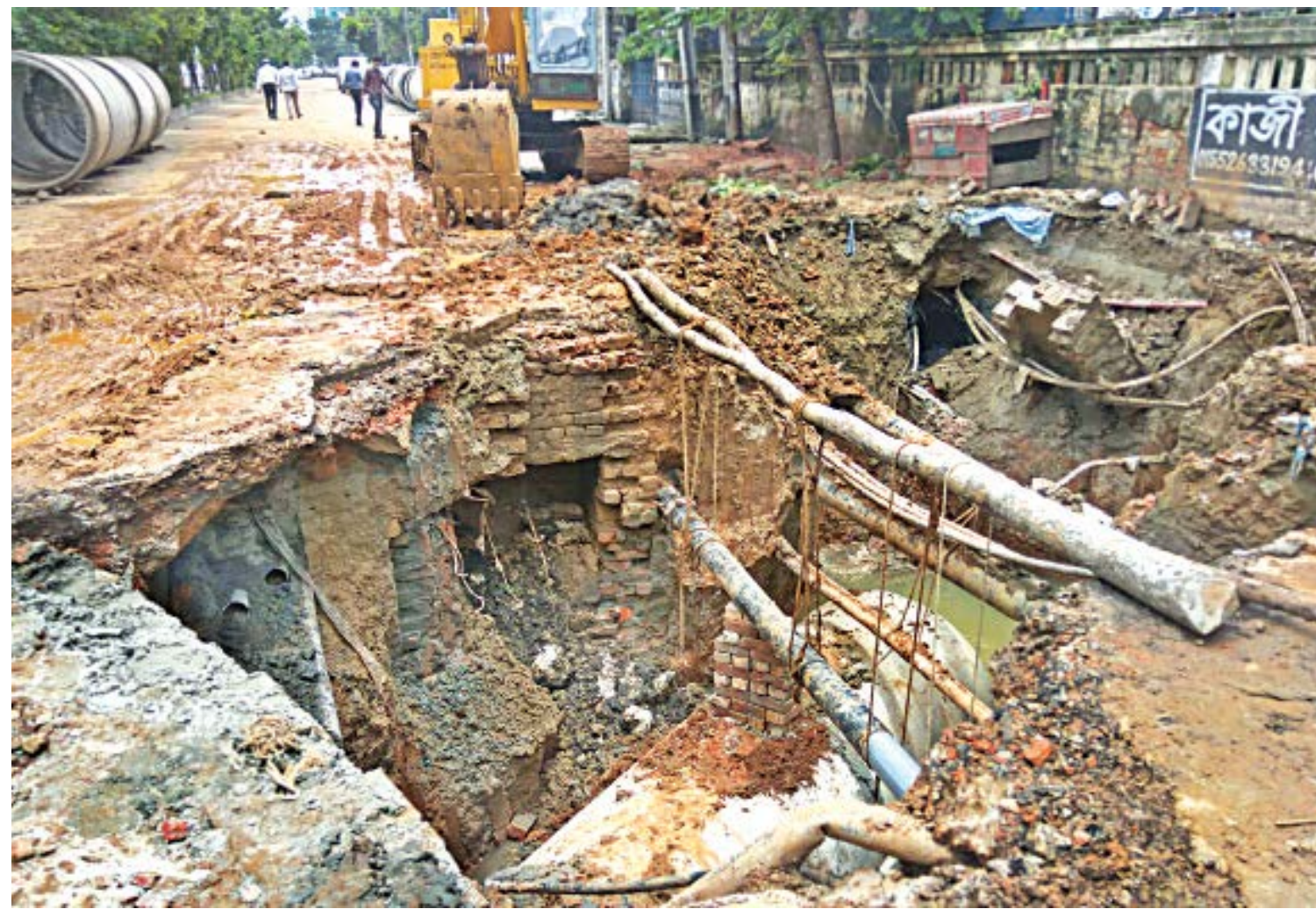
Tying pipes and cables of different utility services to bamboos, Dhaka South City Corporation is installing underground sewerage pipes to widen the lines at Dhanmondi-27. Locals allege that they are suffering immensely as the work progresses slowly. Rainwater also adds to their woes. The photo was taken yesterday.
