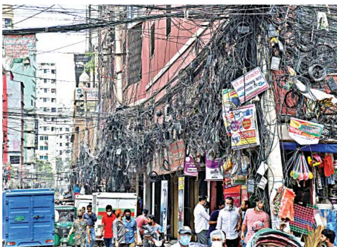
City residents are so used to seeing their roads entangled in overhead cables, many never give a second thought while looking above. But a camera pointed at the madness shows just how severe the mess is. On many occasions, authorities have tried to get rid of this menace, but to no avail. This photo was taken yesterday from the capital's Fakirapool.
