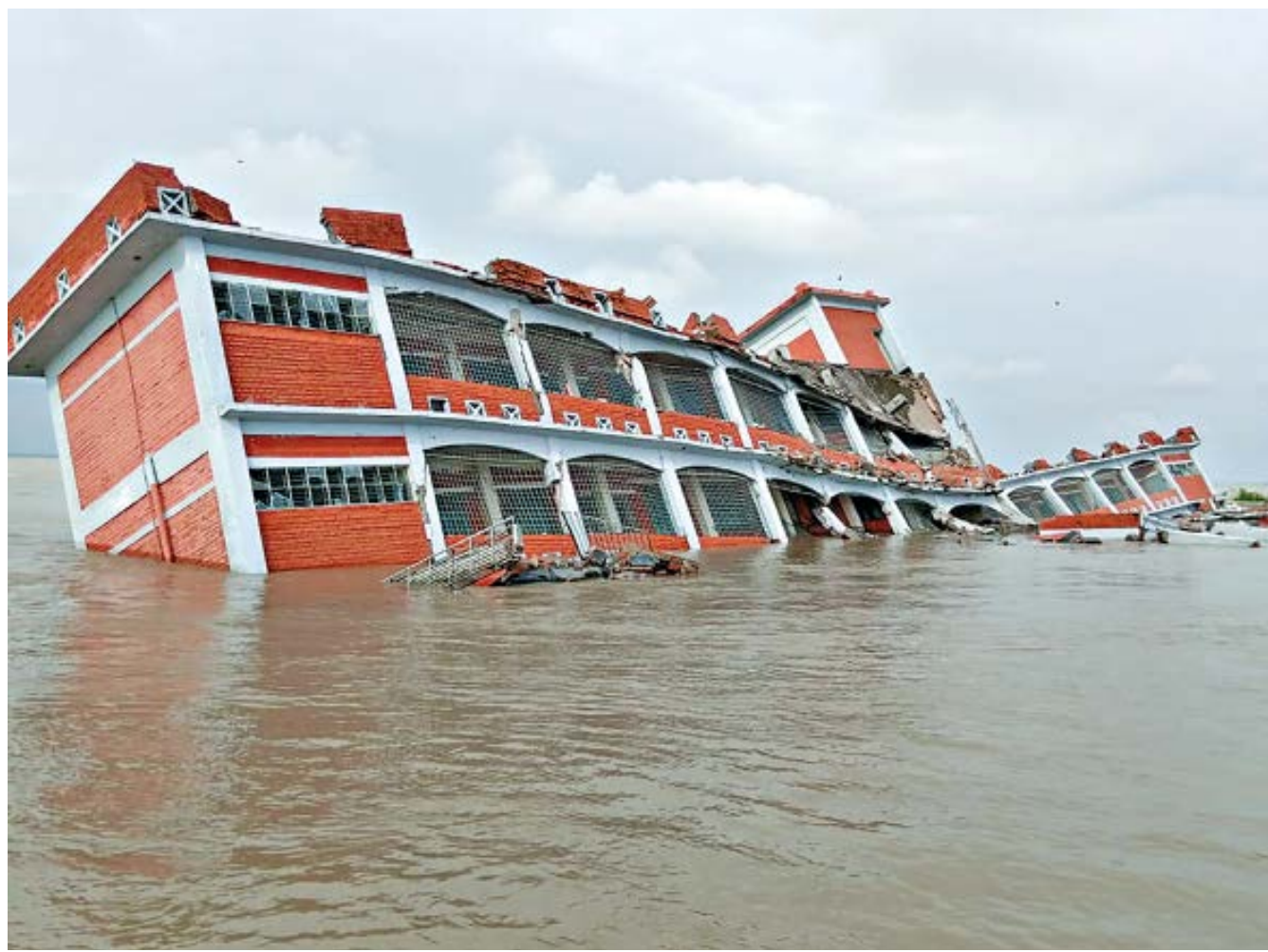
The three-storey building of Nuruddin Matborerandi Model High School is warped out of shape as the ground on which it stood is being washed away by the Padma. The building was barely visible soon after the photo was taken around 5:30pm yesterday in Bandarkhola union of Madaripur's Shibchar upazila. When schools reopen, students of at least 24 villages will have to travel to schools far away from their homes.
