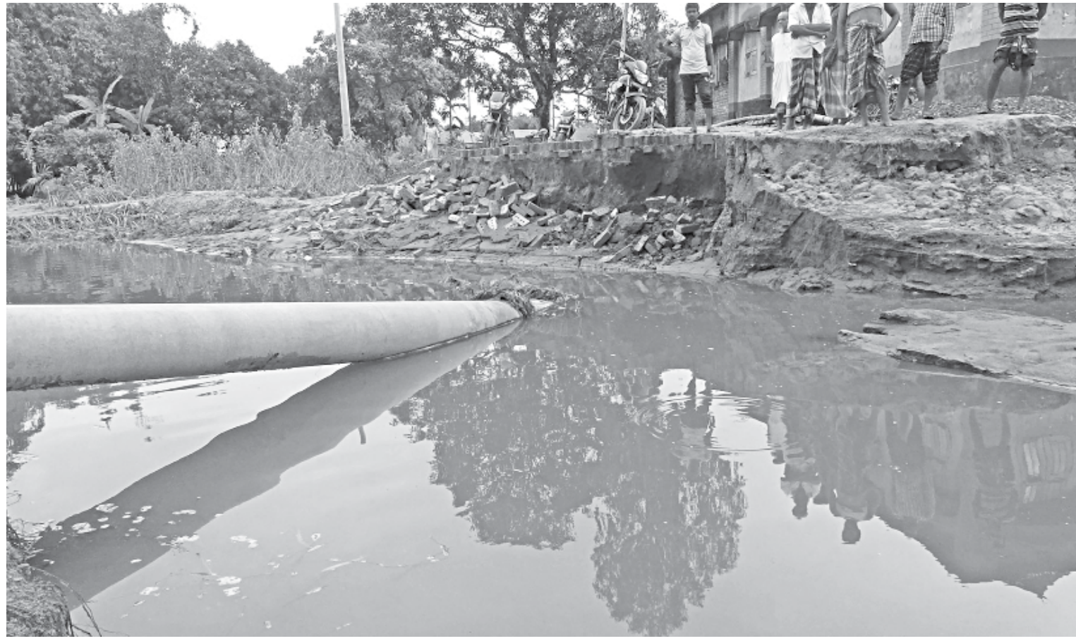
A flood-ravaged road in Dahagram union under Lalmonirhat's Patgram upazila.
