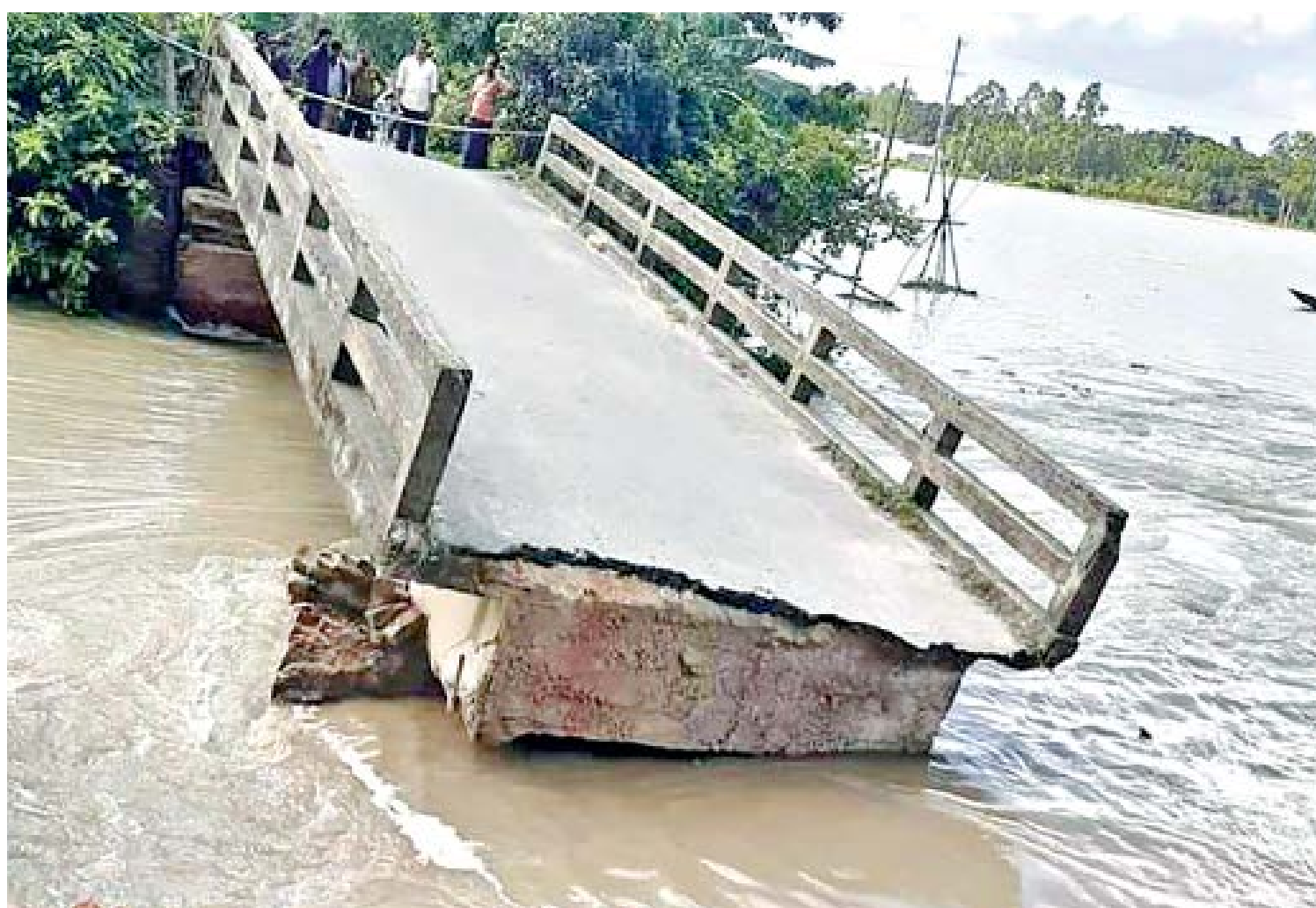
A bridge on Basail-Mirzapur road collapses due to strong currents of floodwater, snapping communications between parts of the two upazilas in Tangail. Six out of the district's 12 upazilas are hit hard by flood which has affected about 1.3 lakh people so far. The photo was taken in Basail's Kanchanpur village on Thursday.
