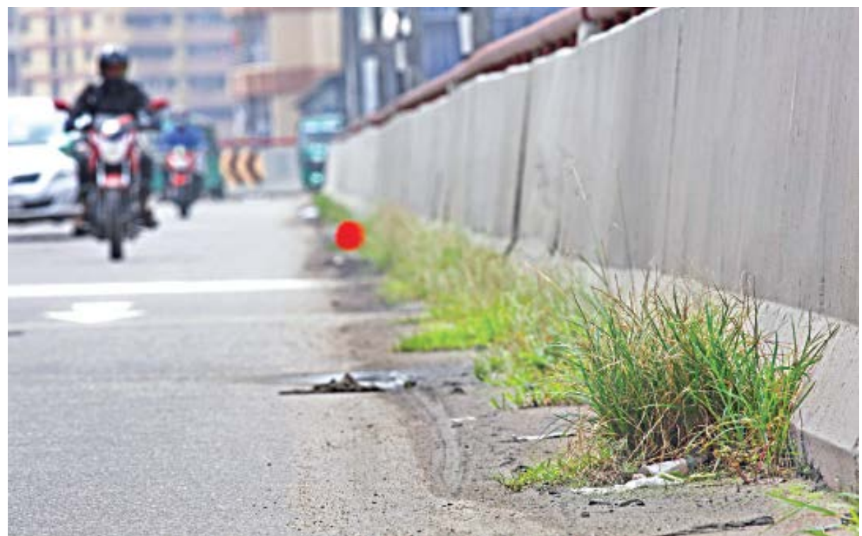
A rather steady stretch of grass growing on a side the Moghbazar flyover makes for an oddly fascinating sight. A combination of factors -- the road remaining somewhat traffic-free during the last few months, possible lack of maintenance and cleanup, and the recent rain -- has created small mud beds on the sides on which the vegetation has sprouted, reminding us that nature can prevail on the most lifeless of manmade creations, given enough time. The photo was taken yesterday.
