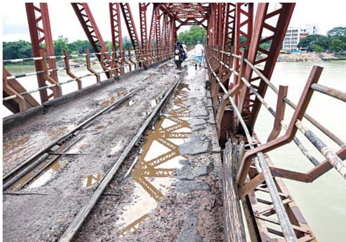
A serious accident is just a matter of time on the run-down Kalurghat Bridge in Chattogram, constructed in the British era. Hundreds of vehicles, plying the bridge, are facing difficulties every day, as the deck and iron fencing on both sides of the bridge have become worn-out and numerous potholes developed on it, giving way to mishaps. Under the circumstances, the railway authorities have decided to suspend vehicular movement on the bridge from 10pm to 8am til July 23 for the much-needed repair work. This photo was taken yesterday.
