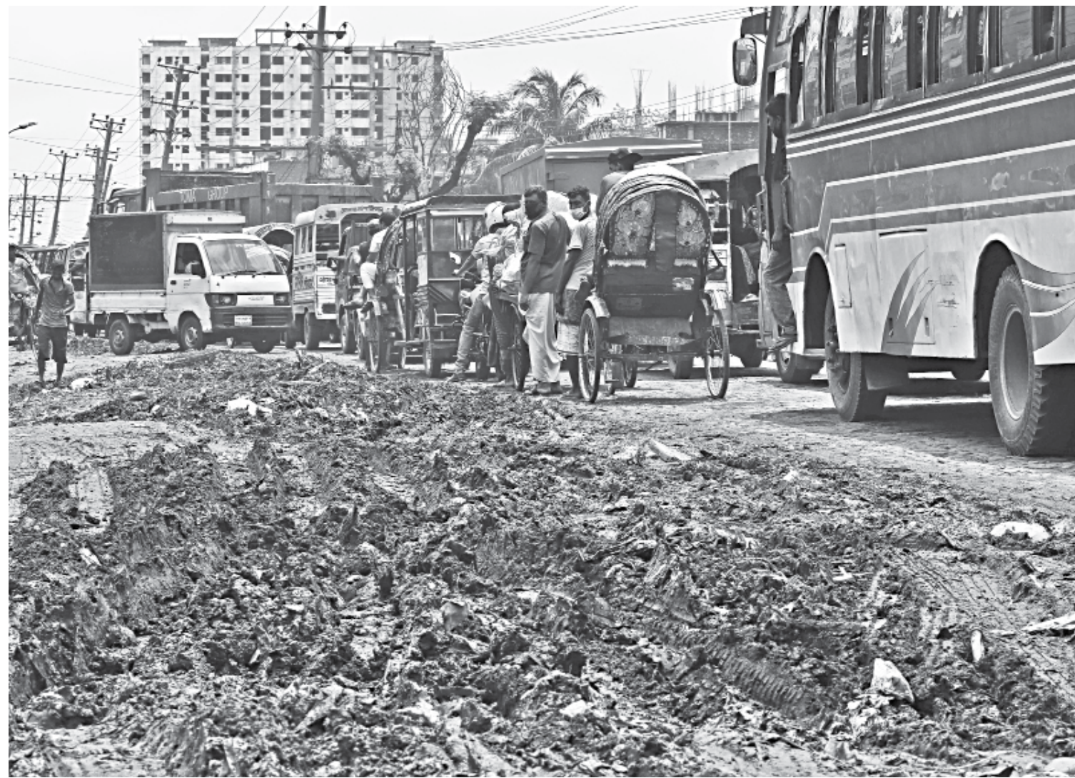
An entire lane of this road in Kajla, Jatrabari has become too muddy for vehicles to pass through, resulting in heavy congestion on the rest of the road. Vehicles are often having to take the wrong side of the road to pass this part, where repair work was ongoing before the rain created a whole swamp. The photo was taken recently.
