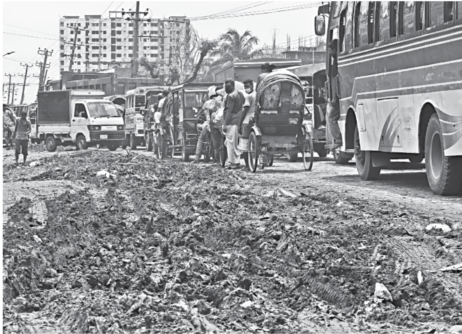
An entire lane of this road in Kajla, Jatrabari has become too muddy for vehicles to pass through, resulting in heavy congestion on the rest of the road. Vehicles are often having to take the wrong side of the road to pass this part, where repair work was ongoing before the rain created a whole swamp. The photo was taken recently.
