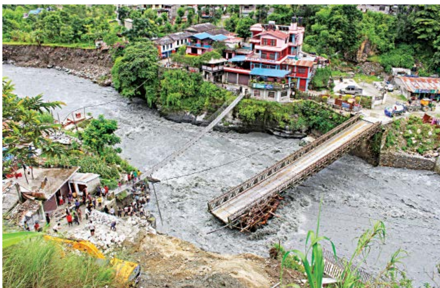
People gather near the bridge that is damaged due to the flood at Raghu Ganga River in Myagdi, Nepal, yesterday.
