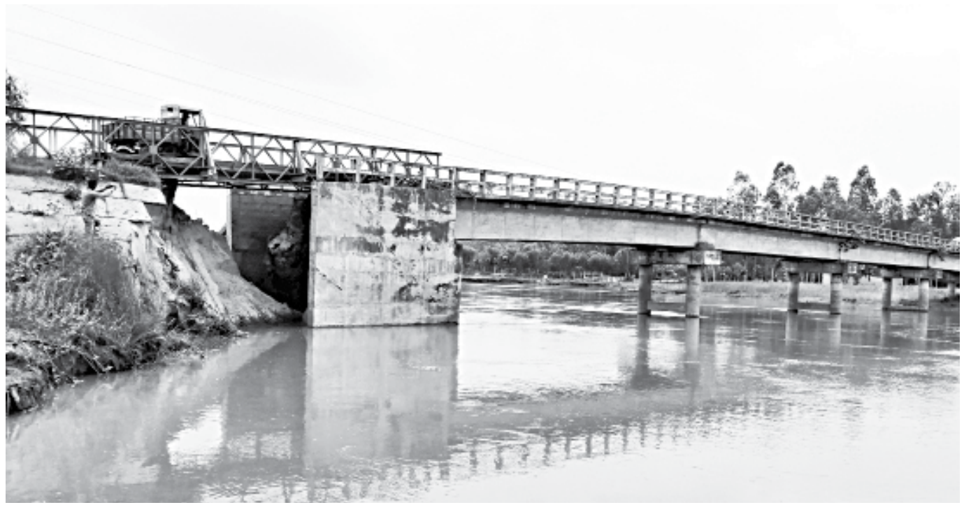
One of the approach roads of the bridge on the Dhaleswari river at Charabari in Tangail Sadar upazila lies badly damaged after the heavy rain for the last several days.
