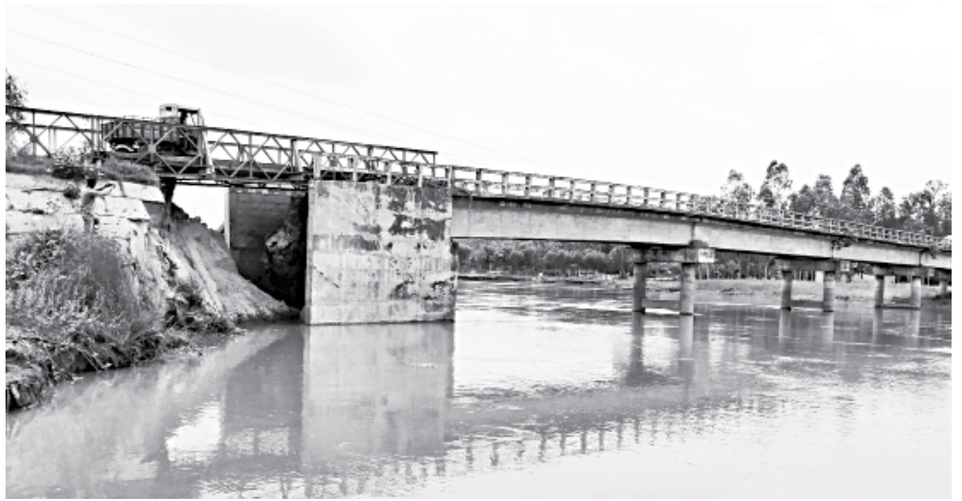
One of the approach roads of the bridge on the Dhaleswari river at Charabari in Tangail Sadar upazila lies badly damaged after the heavy rain for the last several days.
