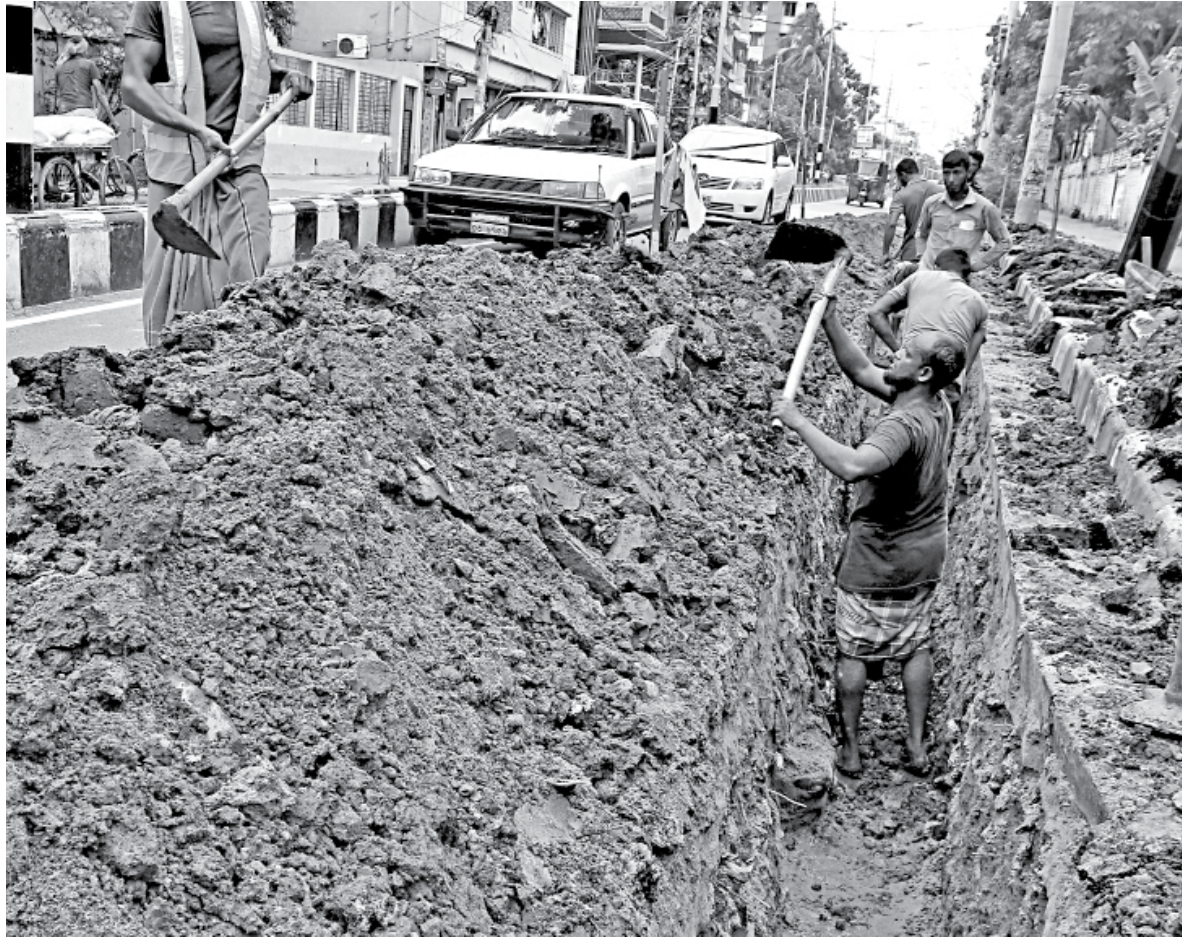
Dhaka Electric Supply Company (Desco) has chosen an inopportune time to dig up this road in Mirpur-1 for work on underground cable lines, as rainy weather may not just slow the work down but also pose hassles to commuters. Locals said the road was renovated just a year ago and was in perfectly good shape until the excavation. The photo was taken yesterday.
