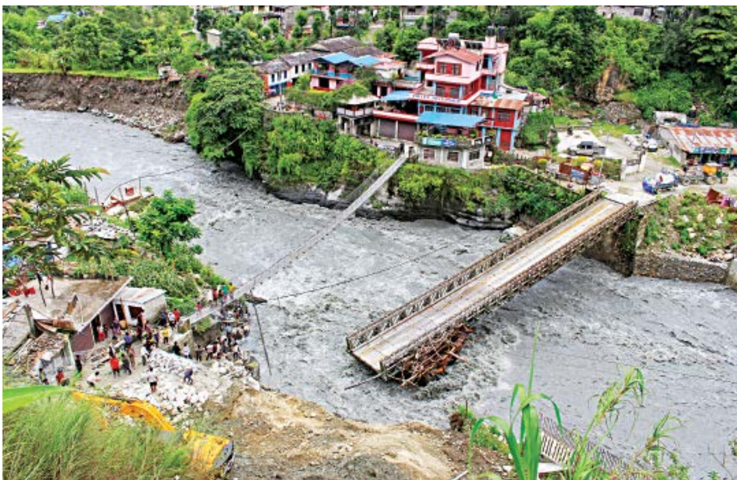
People gather near the bridge that is damaged due to the flood at Raghu Ganga River in Myagdi, Nepal, yesterday.
