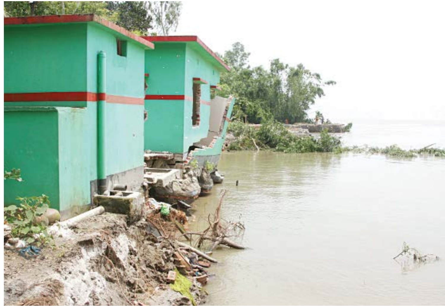
A concrete building being slowly devoured by the Jamuna at Beltia village of Tangail's Kalihati upazila. At least 40 such structures, mostly homes, have been washed away over the last couple of days after erosion damaged a portion of the flood protection embankment in the area. The villagers have blamed the Water Development Board's negligence in this regard. The photo was taken yesterday.
