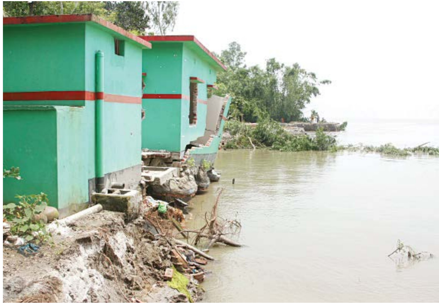
A concrete building being slowly devoured by the Jamuna at Beltia village of Tangail's Kalihati upazila. At least 40 such structures, mostly homes, have been washed away over the last couple of days after erosion damaged a portion of the flood protection embankment in the area. The villagers have blamed the Water Development Board's negligence in this regard. The photo was taken yesterday. PHOTO: MIRZA SHAKIL
