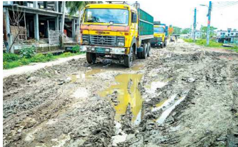
Bituminous surface has totally disappeared from Bastuhara bypass road in Khulna. The photo was taken recently.
