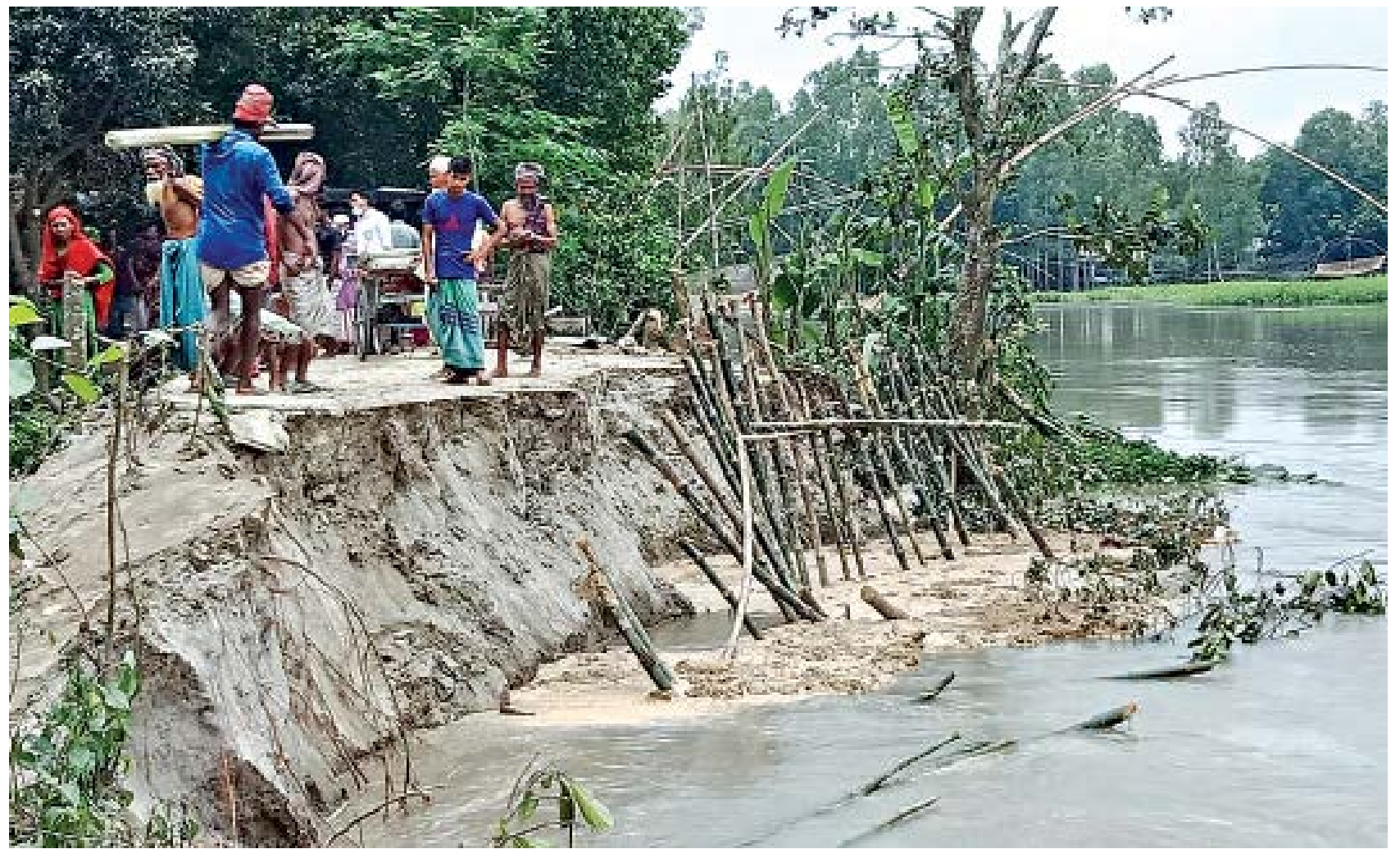
The swelling Jamuna devouring a flood protection embankment at Shubhogachha village in Sirajganj's Kazipur upazila yesterday. People who live near the embankment have started dismantling their homes and moving elsewhere fearing that they would be marooned or their homes destroyed.
