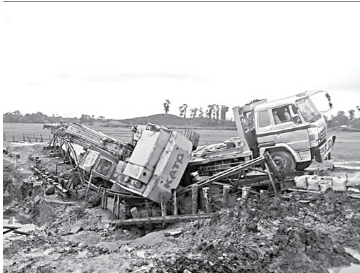
Road communication between Fultola and the upazila headquarter remains suspended since Friday morning after an under construction Bailey bridge on a diversion road collapsed at Kapnapahar in Moulvibazar's Juri upazila.
