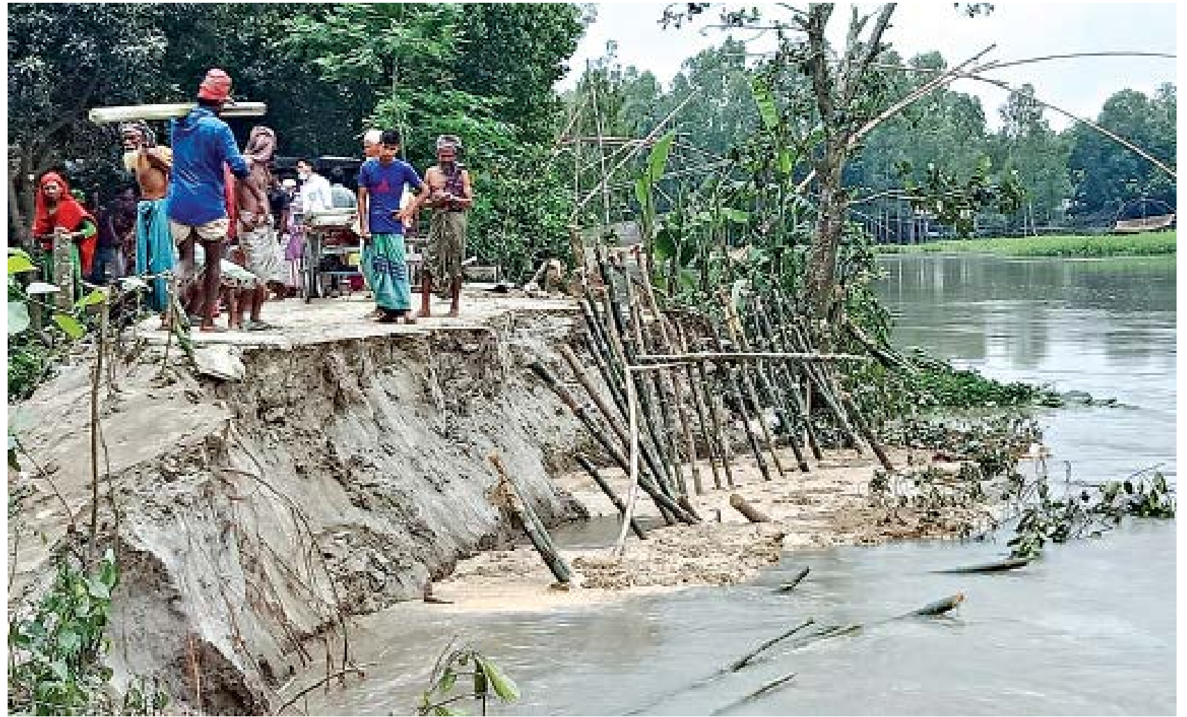
The swelling Jamuna devouring a flood protection embankment at Shubhogachha village in Sirajganj's Kazipur upazila yesterday. People who live near the embankment have started dismantling their homes and moving elsewhere fearing that they would be marooned or their homes destroyed.
