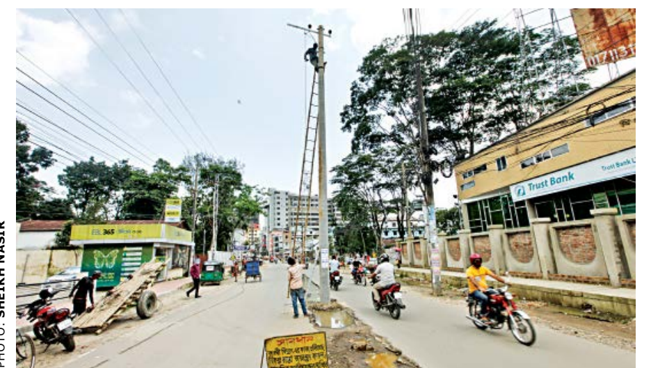
BPDB is installing electric poles in the middle of the roads from Amberkhana to Bandarabazar, for streetlights and a backup for the underground power lines.
