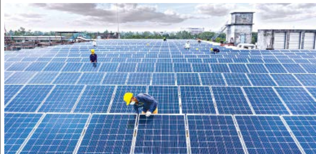
A view of the solar panels installed on the roof of Square Textiles in Gazipur. The company plans to expand its renewable energy use.
