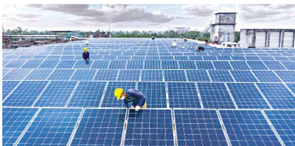
A view of the solar panels installed on the roof of Square Textiles in Gazipur. The company plans to expand its renewable energy use.
