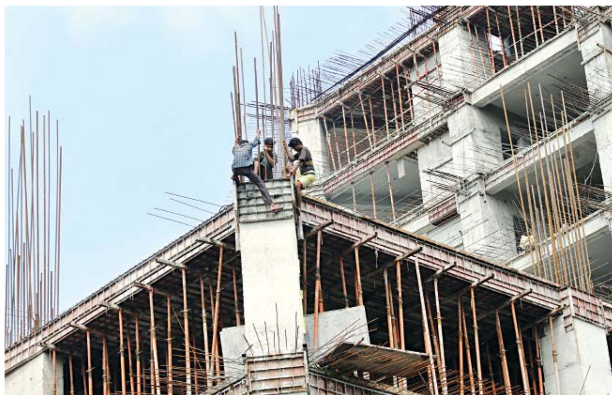
Without wearing any safety gear, labourers work at an under construction building in the capital's Tejgaon industrial area yesterday. They do not even have any masks on. One could get fined for not wearing a mask.
