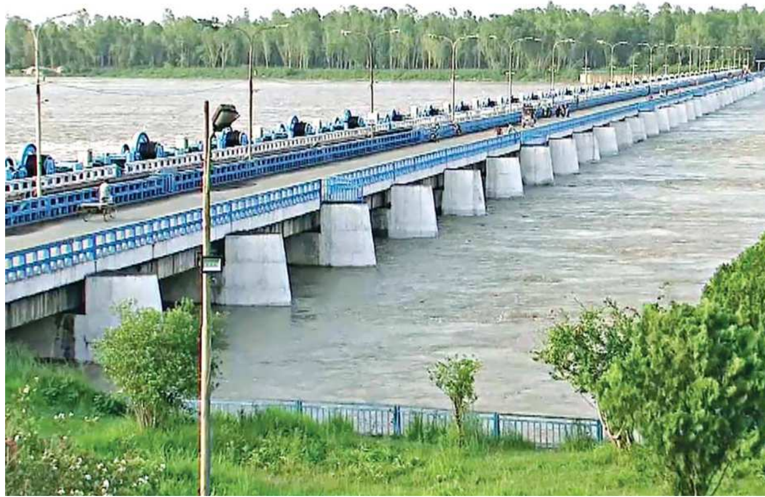
Water rushes through the Teesta Barrage over the danger level at Hatibandha upazila of Lalmonirhat yesterday. Water levels of several other rivers in the country are also rising.
