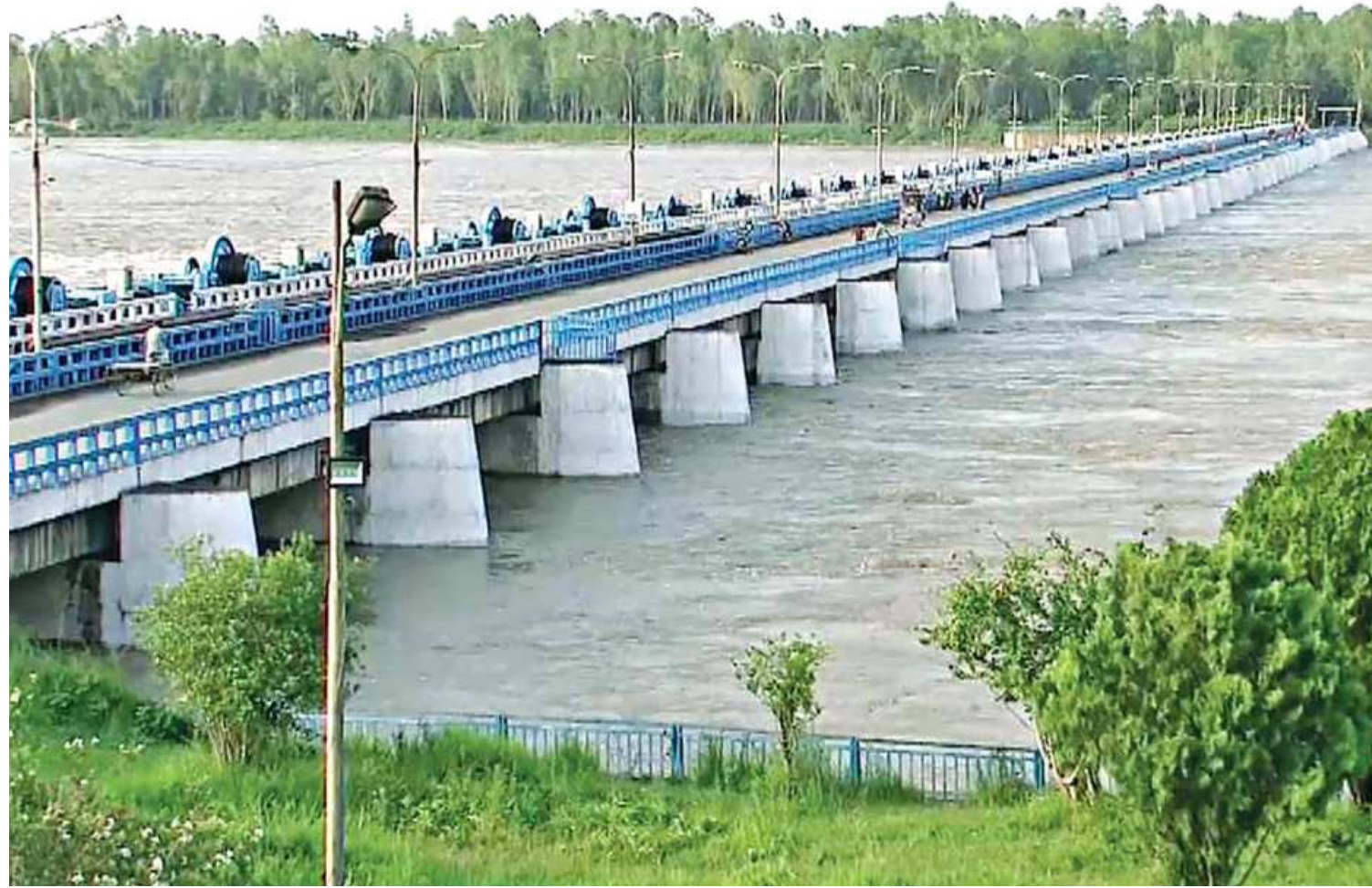
Water rushes through the Teesta Barrage over the danger level at Hatibandha upazila of Lalmonirhat yesterday. Water levels of several other rivers in the country are also rising.
