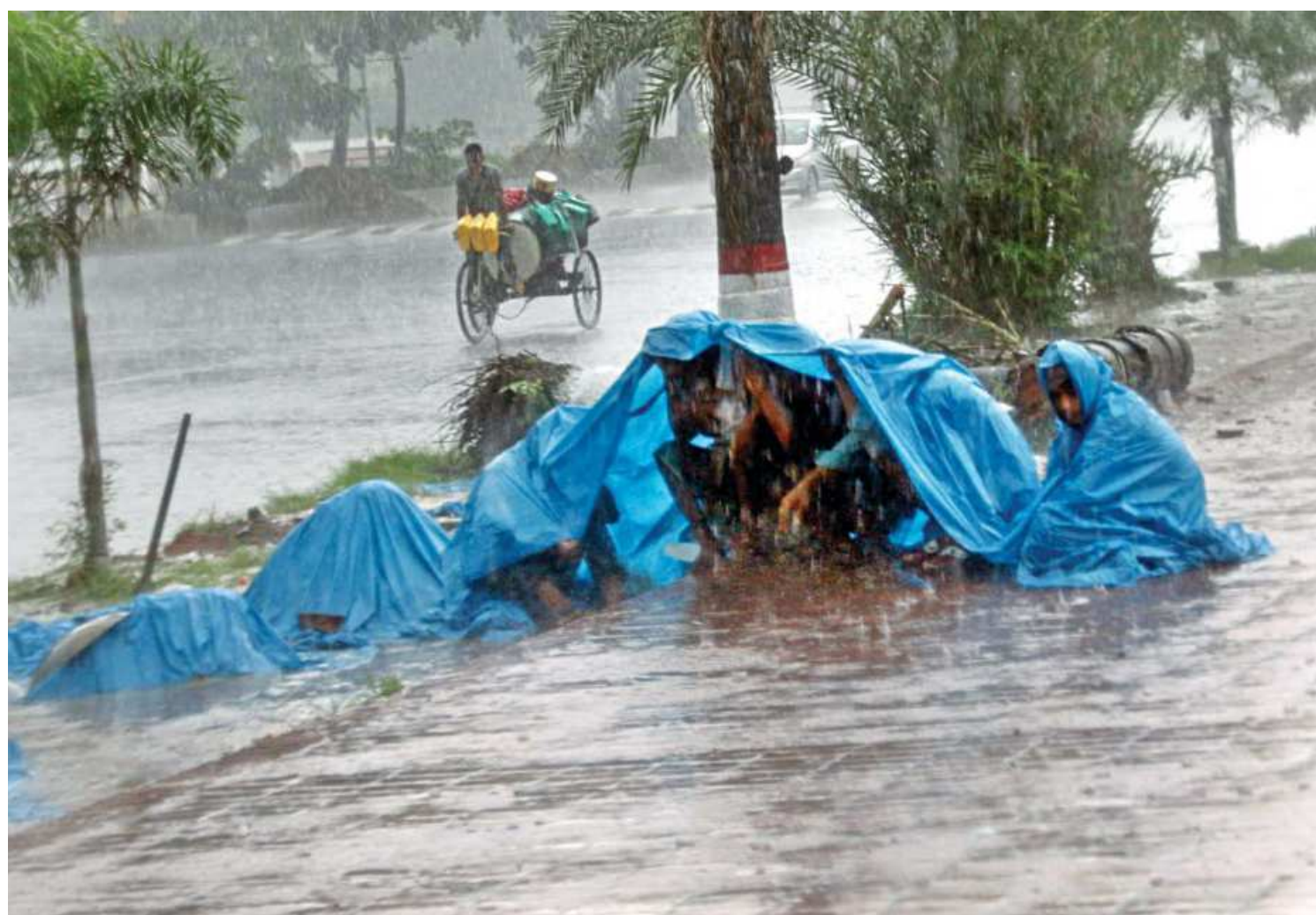
Workers who were repairing a part of the capital's Manik Mia Avenue take shelter under a polythene sheet amid sudden rain. Light rain in parts of the city caused sufferings to day labourers yesterday.
